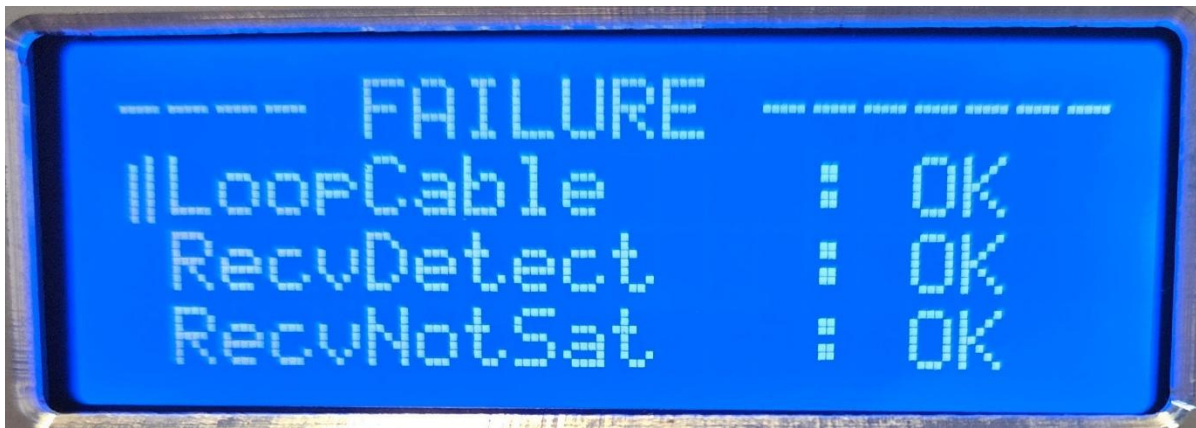
Figure 62. Front panel display – failure LoopCable, RecvDetect, RecvNotSat
